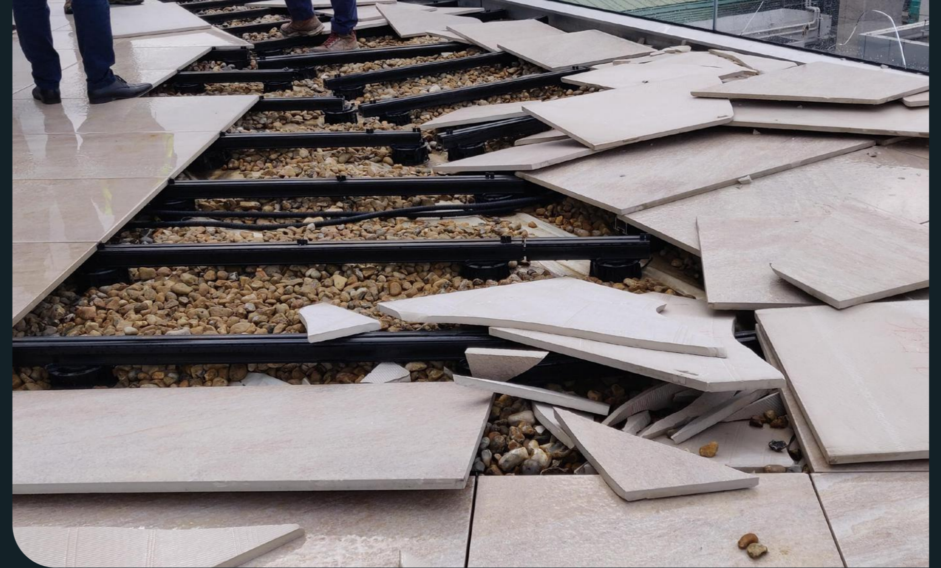
Tiles on a roof terrace which have been damaged by wind uplift.
